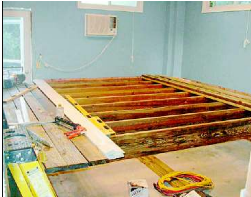
Once the permit was approved, we started work on the most critical part of the project — raising the floor to meet FEMA minimum flood requirements. The door to the outside (left) was raised next.
